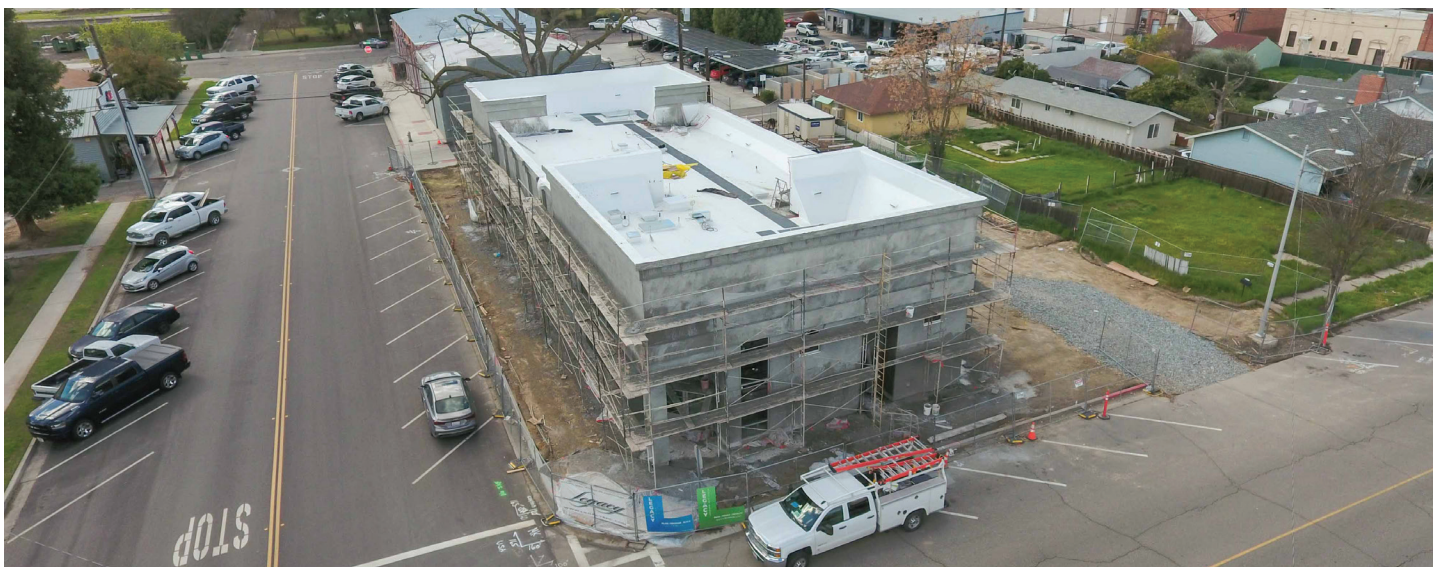
The Fowler Health Center is under construction. Its completion is anticipated for Winter 2023.
